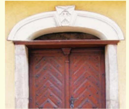
Stone portal and the door made of floorboards in the house standing at 47 Stojalowskiego Street, dating back to the turn of the 18th and 19th centuries. Apart from floorboards arranged in herringbone and lozenge pattern, the door is embellished with a column-like astragal.
