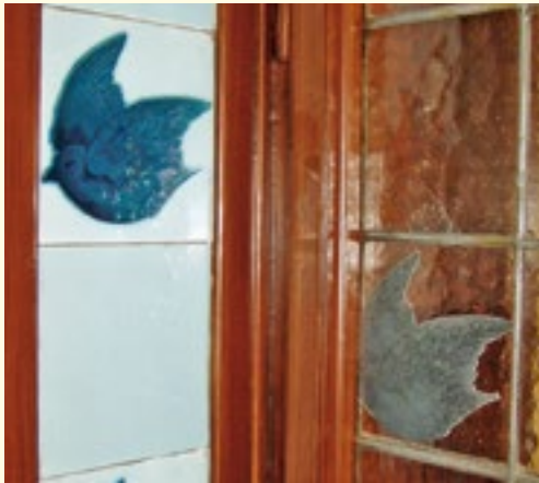
Ceramic cladding of the window recess with an image of a pigeon and a fragment of a stained glass window with the same motif – elements of Art Nouveau interior decorations of the villa of Emanuel Rost, Jr. at 48 Komorowicka Street.
