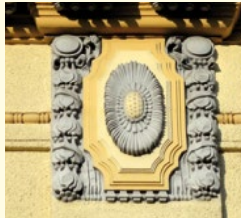
A fragment of stucco decorations on Franciszek Polaczek's residential house at 5 Barlickiego Street. This early modern house was put up in 1910 by a partnership of architects Georg Weinzettel & Wilhelm Riedel.
