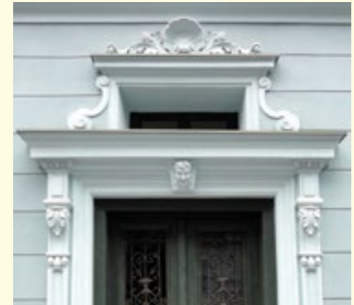
Neo Baroque framing of the door and a decorative lintel with a fanlight above in a building that used to belong to the Morawitz family, situated on the corner of 23 Rynek and 1 Wzgórze Street. In the doorway forged grating made of cast iron.
