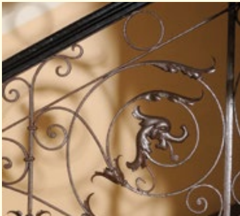
Forged cast iron balustrade with a subtle motif of acanthus leaves, adorning the staircase in Victor Burda's residential house at No. 10, 11 Listopada Street, designed by Karl Korn.
