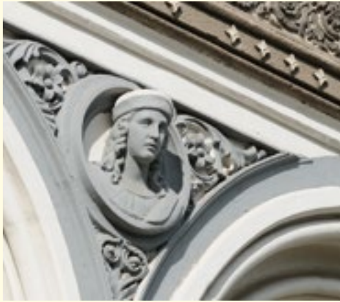
Neo-renaissance stucco decorations embellishing the front façade of the former Protestant Teacher's College at Plac Lutra 8 (8 Luther's Square), erected by Emanuel Rost, Sr. in 1863.
